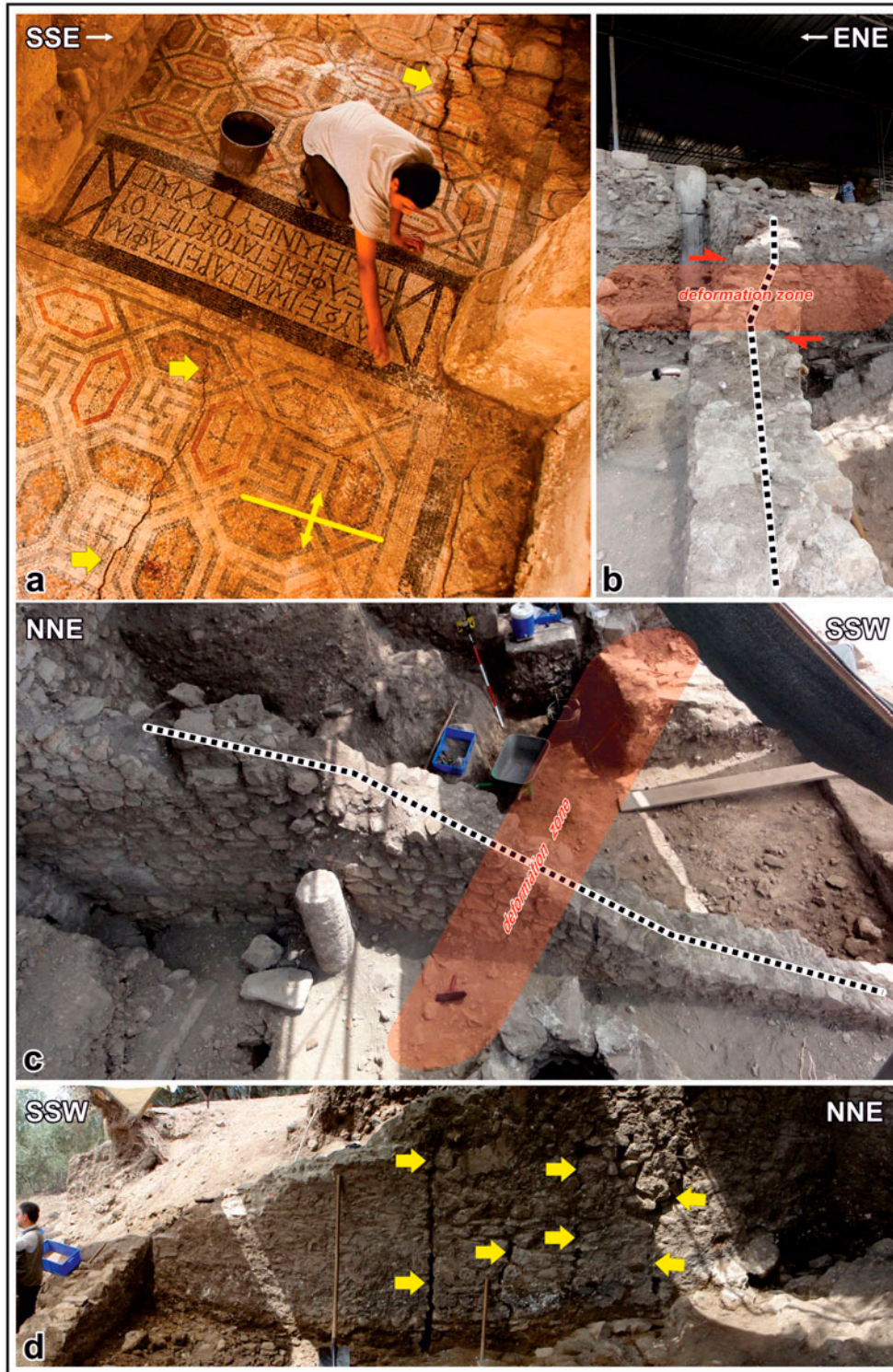
Figure 8. (a) Extensional cracks and undulations observed on the floor (yellow arrows) of Apodyterium of the Roman villa (photo taken from www.antandros.org ). (b and c) E–W directed dextral shear zone (red shaded area) on the ancient wall, dotted line indicates rotation geometry. (d) Systematic E–W trending cracks and fractures (yellow arrows) observed in the western wall. Persons for scale in all photos are 1.75-m long.
