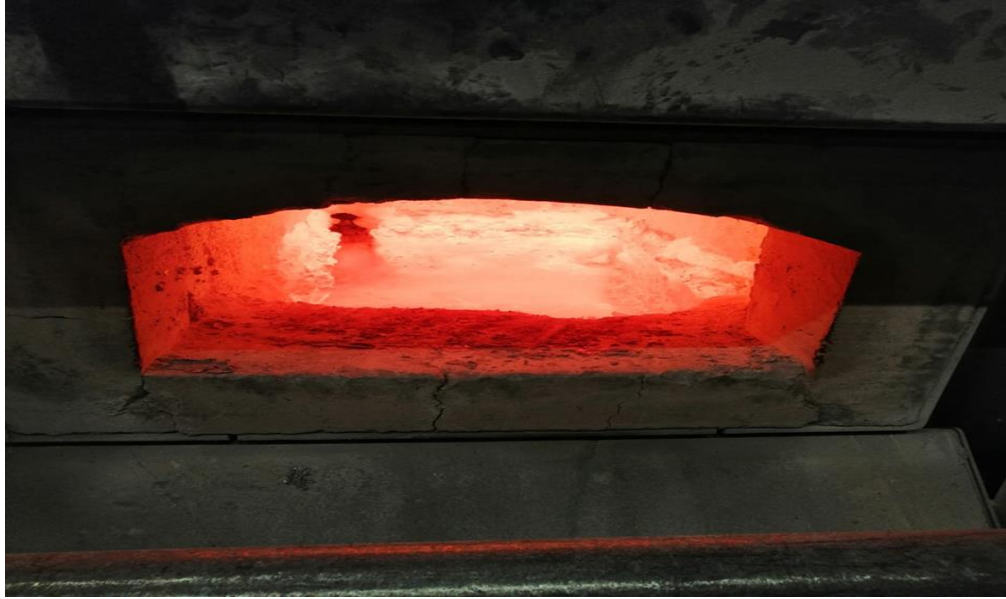
Figure 4.1 Example of corrosion on edge walls in aluminium melting furnace (Personal archive, 2020)
